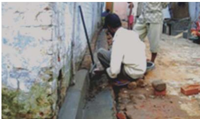
The intervention enabled people to get small drains constructed in front of their houses which are linked to the big drain
